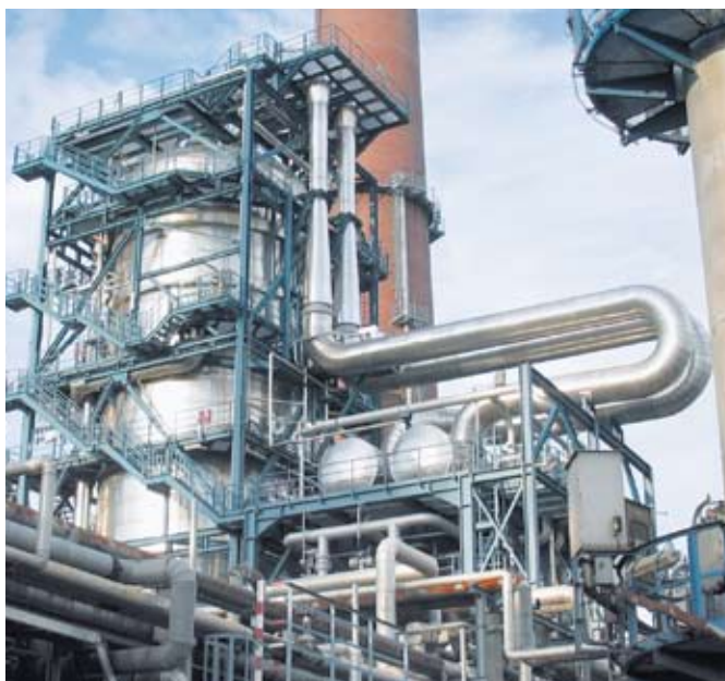
Fig. 4 3-stage steam jet vacuum pump with surface condenser for the vacuum column of a refinery Suction flow: 13 180 kg/h (436 000 m 3 /h) Suction pressure abs.: 4.5 kPa abs. Discharge pressure abs.: 110 kPa abs.
