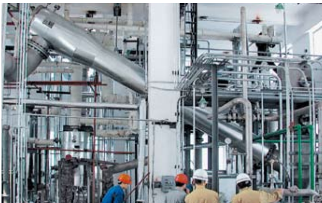
Fig. 3 3-stage steam jet vacuum pump with mixing condenser and liquid jet vacuum pump in a polyester production plant
