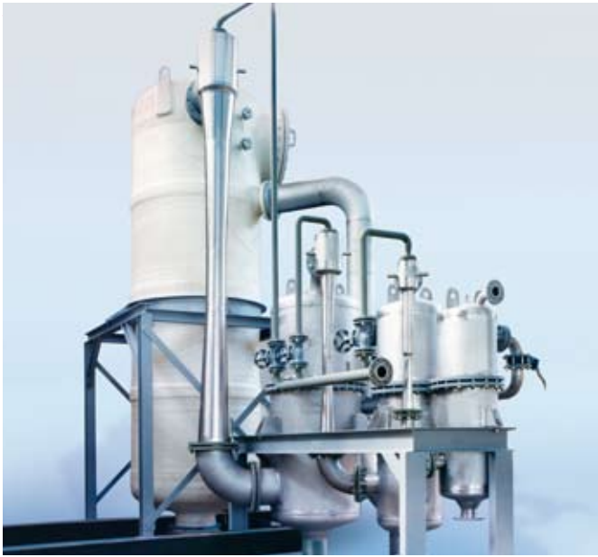
Fig. 2 3-stage steam jet vacuum pump with mixing condensers Suction capacity: 3380 kg/h steam and 225 kg/h of inert gas from 60 mbar
